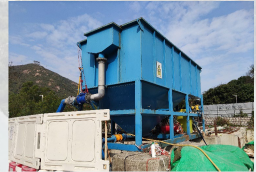
Wastewater treatment facility
